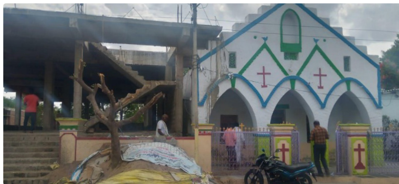
Construction of the new building for the MB church in Volluru Village
